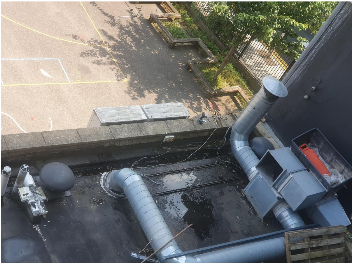
Figure 5 - Image showing new location of Simmons Bar's fans, to help with reduction of noise impacting residents.
